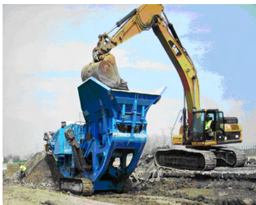
Concrete pavement being recycled on site with portable crushers for reuse in new pavement section on the South Tri-State (I-294)
