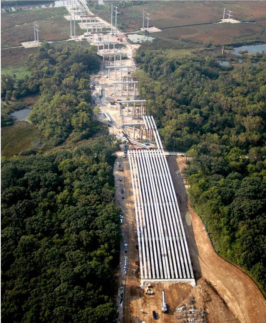
The Des Plaines River Valley Bridge begins to take form as construction continues on the I-355 South Extension Project.
