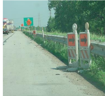
Remove unused devices
