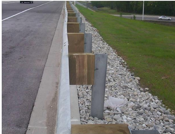
Figure 9.0 Midwest Guardrail System
