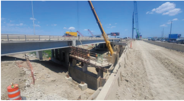
Roadway and bridge reconstruction is underway along the Central Tri-State Tollway (i-294) as part of the I-490/I-294 Interchange Project near Franklin Park.
