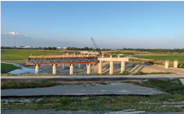
Bridge piers are constructed along the Jane Addams Memorial Tollway (I-90) as part of the I-490/I-90 Interchange near Des Plaines.
