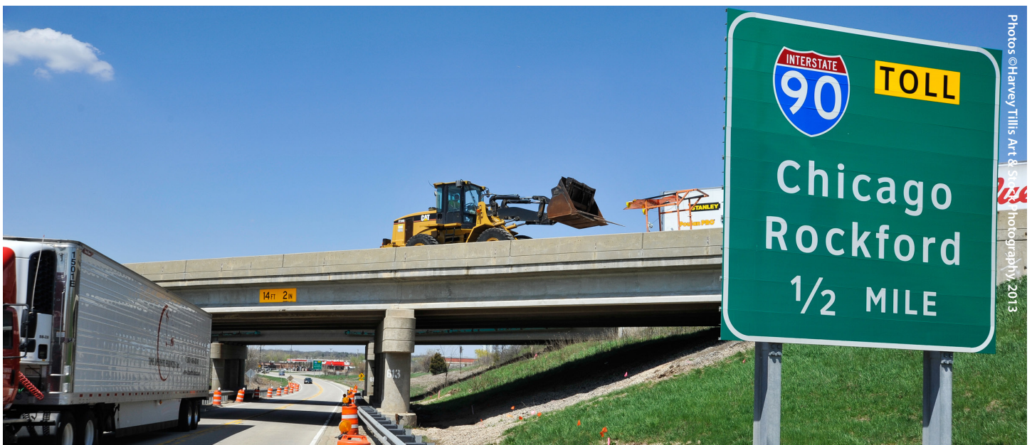
Acura prepares to begin rebuilding and widening work on the U.S. Route 20 Bridge on the Jane Addams Memorial Tollway (I-90) near Hampshire.
